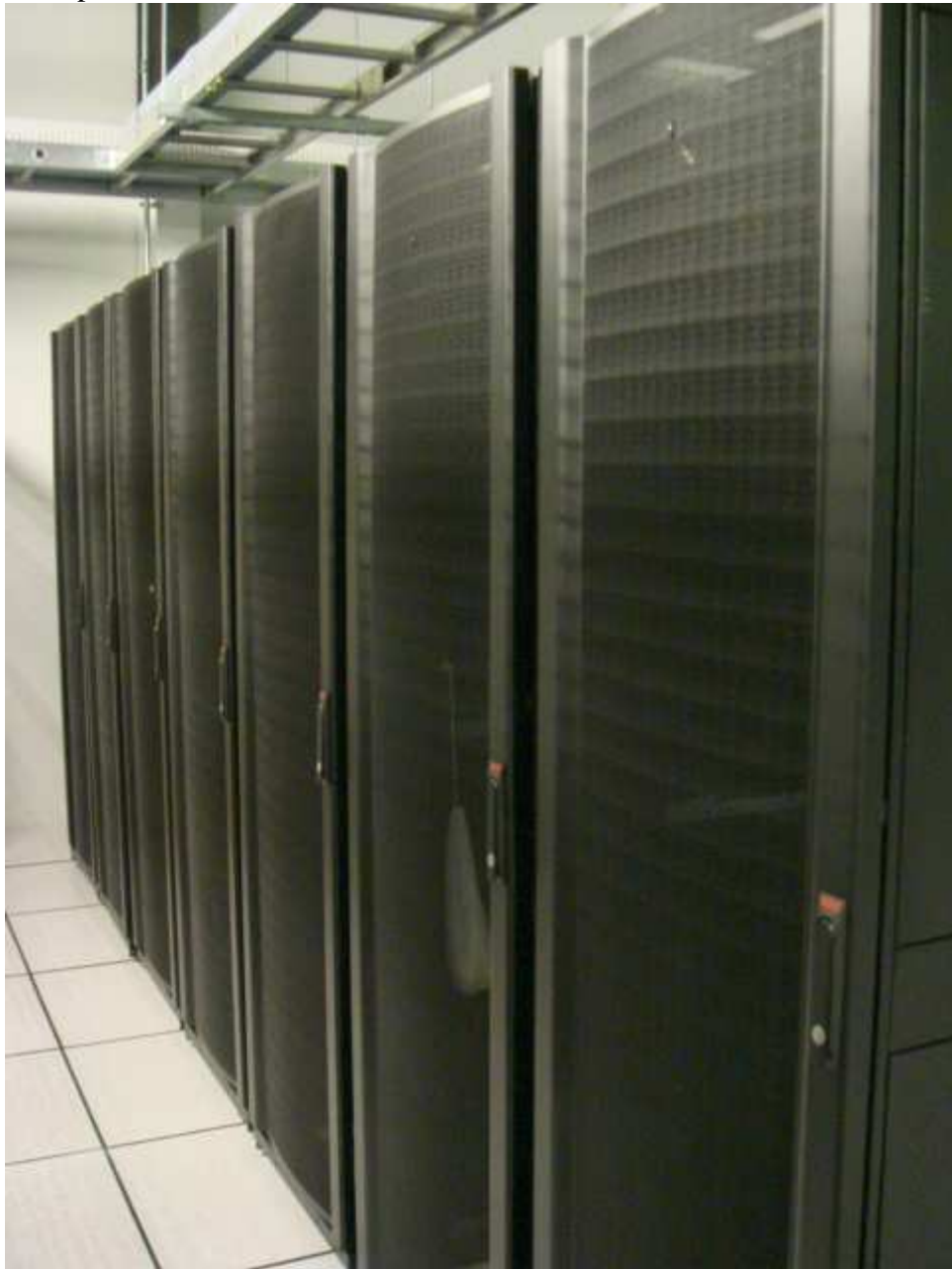
Example of a Hot / Cold aisle
